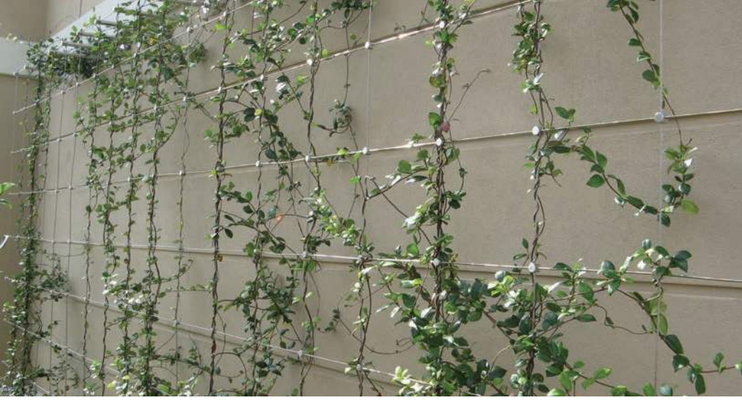
ABOVE: CARL STAHL DECOR CABLE SYSTEM IN JUPITER, FLORIDA RETAIL SHOPPING CENTER Image provided by: Patrick Kelly
